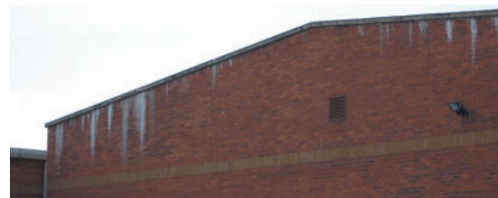
Characteristic lime staining 'runs' from mortar joints
