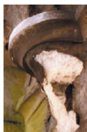
Damage to stonework due to Cryptoflorescence
